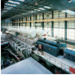
Typical Power Station Turbine Hall where years of experience have been gained working in confined and high cleanliness areas of plant.
