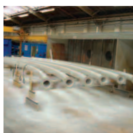
Sulphuric acid tank lining and coating for conventional power station water treatment plant.
