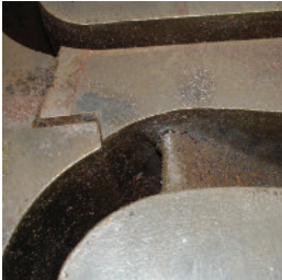
Each of the cast components had cracks as severe as that shown in this photograph.
