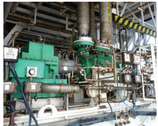
Figure 12. First unit commissioned at site.
