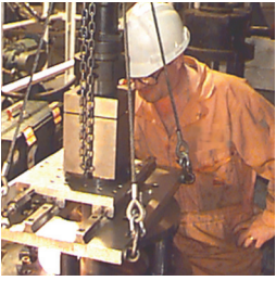
Weir has extensive experience in delivering a proven leak-free valve outage service.
