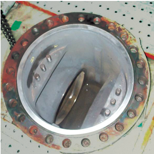
Access to valve seats in-situ often poses challenges.
