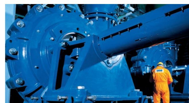
Warman type L centrifugal slurry pumps on FGD absorber recycle duty at the Prunerov Power Station in the Czech Republic
