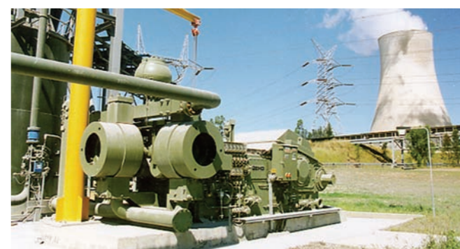
GEHO piston diaphragm pump transporting fly ash slurry from Bayswater Power Station to the Ravensworth Void, Australia
