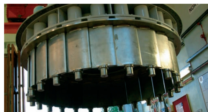
Hydro turbine top cover assembly
